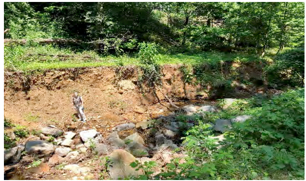
A before picture, above, shows the extensive stream erosion threatening the water main, trail, and trees along the stream channel.
